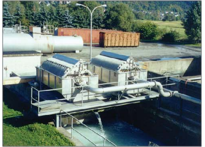
Germany Power generation plant waste water treatment system outlet water filtration
